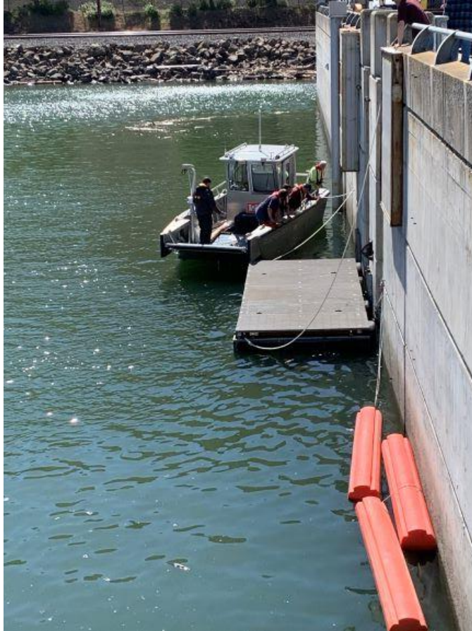
Figure 8. The second, improved temporary debris boom being installed at the south fish ladder exit on May 4, 2021. First debris boom in lower right.
